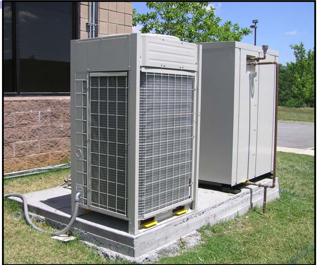
Photograph of the installed system (Daikin IS-VRV™) outside the EPRI Knoxville facility.
