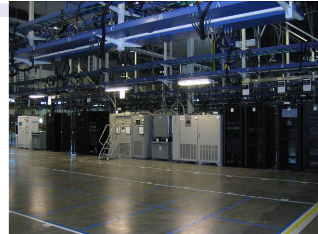
DC Power Distribution
