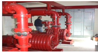
Blowers in a municipal wastewater treatment facility
