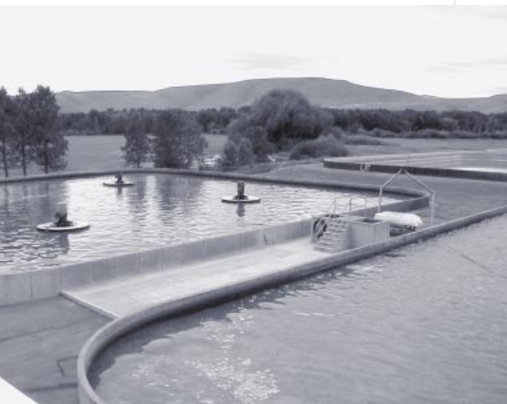
Wastewater Treatment Plant Aeration Basin, Ellensburg Wastewater Treatment Plant, Ellensburg, WA.
