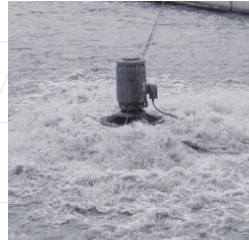
Wastewater Treatment Plant Aerator, Ellensburg Wastewater Treatment Plant, Ellensburg, WA.
