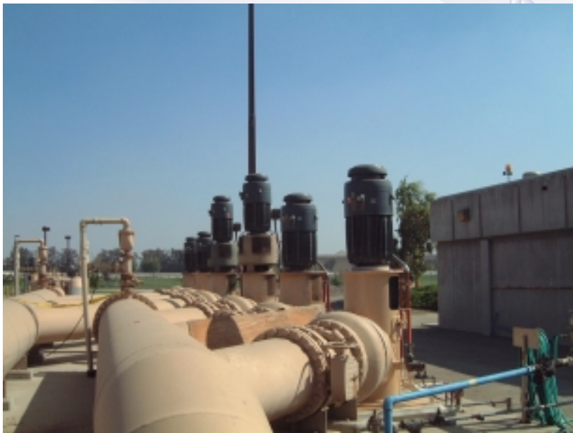
The IPS Pumping System with 6 New Direct-Drive Pumps
