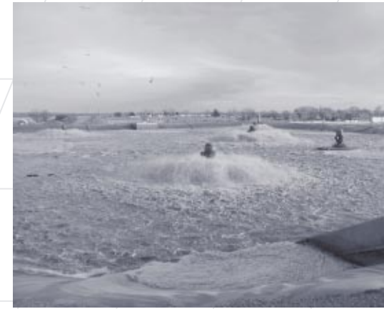
North High Rate Treatment Basin at the Kennewick Wastewater Treatment Plant, Kennewick, WA
